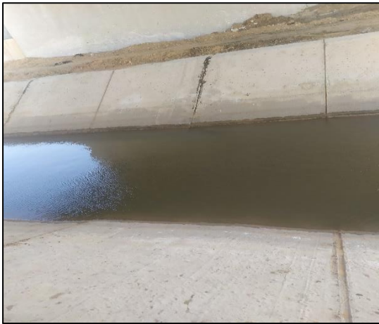
Photo (3): Water seepage into the canal
