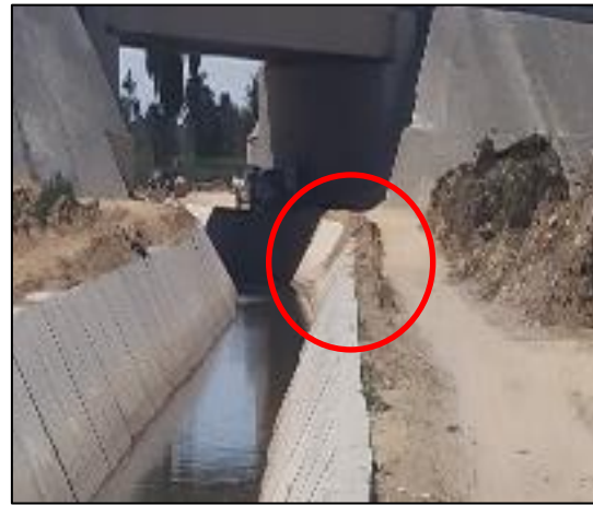
Photo (5): Sliding in some lined slabs
