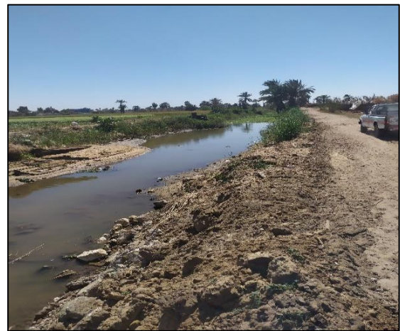
Photo (6): Failure of canal side slopes
