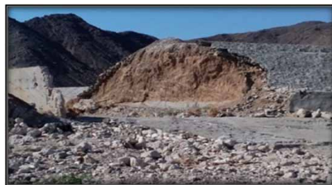
Figure 1 | Subgrade failure of the Qena–Safaga Track due to flooding (Egyptian Railway and Abuzeid et al. 2022).
