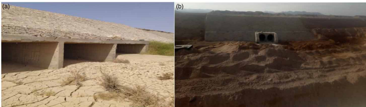
Figure 8 | Examples of sediment accumulation: (a) inside and in front of culverts, and (b) in front of culverts (Egyptian Railway).
