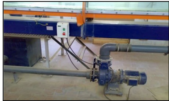
Photo (2): View of the electrically driven pump
