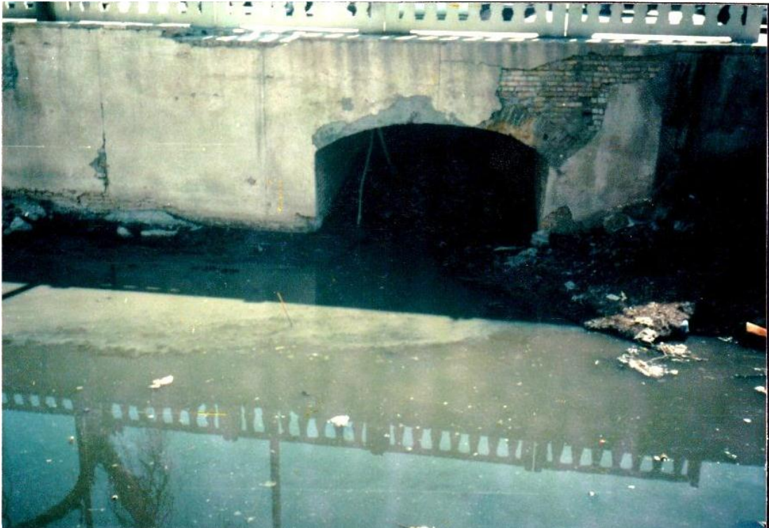
Fig. 2: Ashar branch pollution by discharging pollutants resulting from domestic uses as well as discharging solid waste (garbage) on its sides. 8/11/2015
